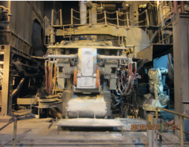
Fig. 5 - SMS automatic slag door Condoor and robot for sampling and measuring inside dog-house at Riva Acciai Caronno
