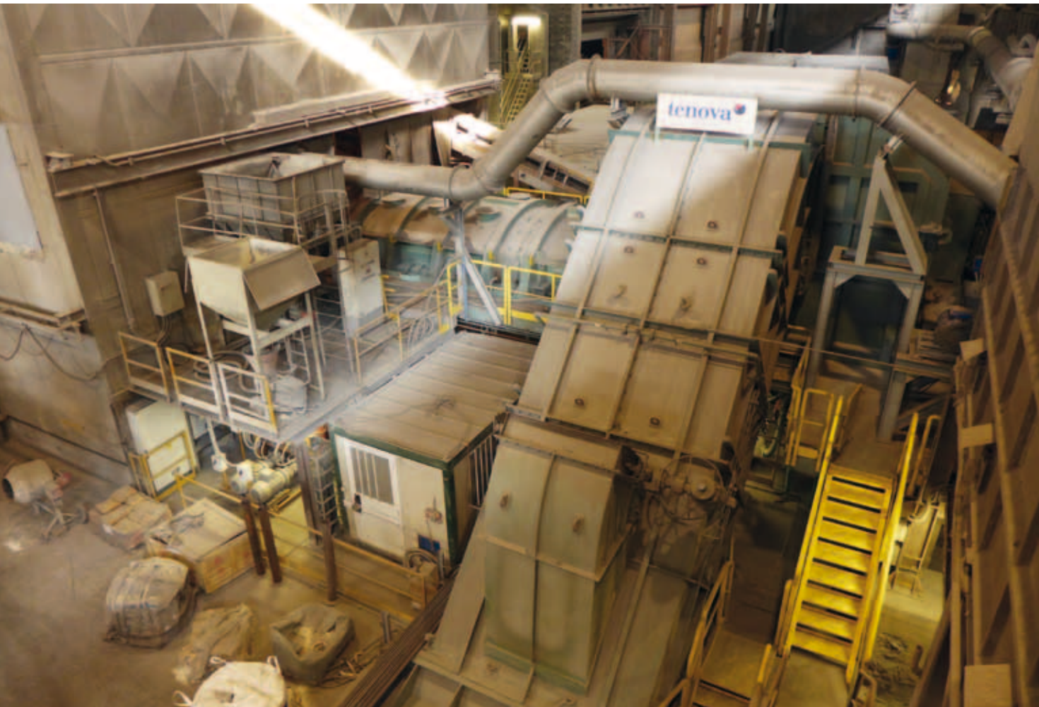
Fig. 3 - The new revamped Consteel ® , offtake hood side.
